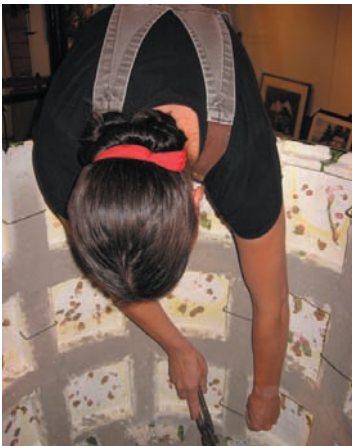
Kacheln are set first with mortar (which is 25% grog and 75% clay) and wire "staples." The flue structure is built inside, layer by layer, from the ground up.
