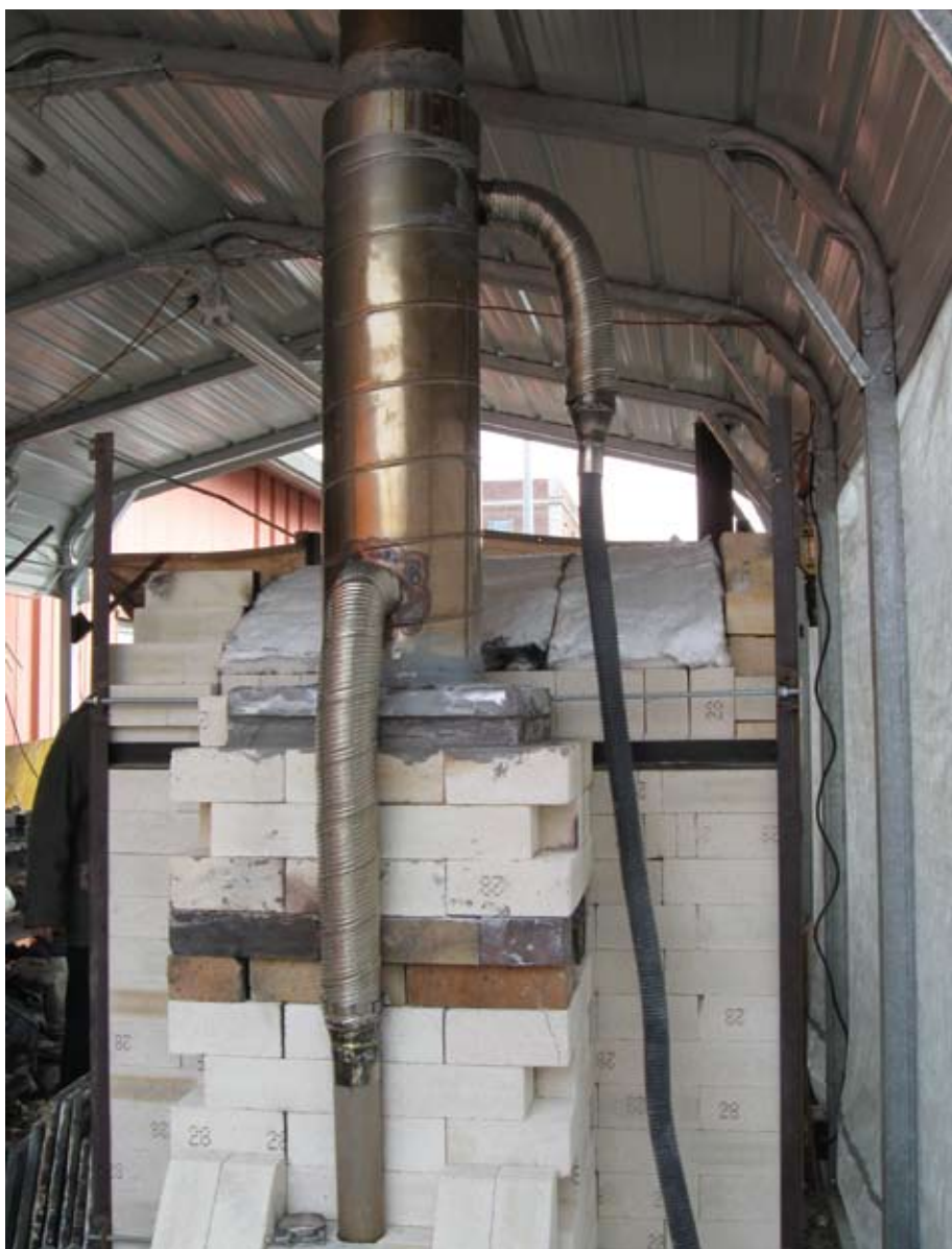
The recuperative chimney on one of Shippensburg University's kilns reclaims heat from the exterior of the chimney and the warm air is used with the drip plate burner system to enhance fuel combustion.
